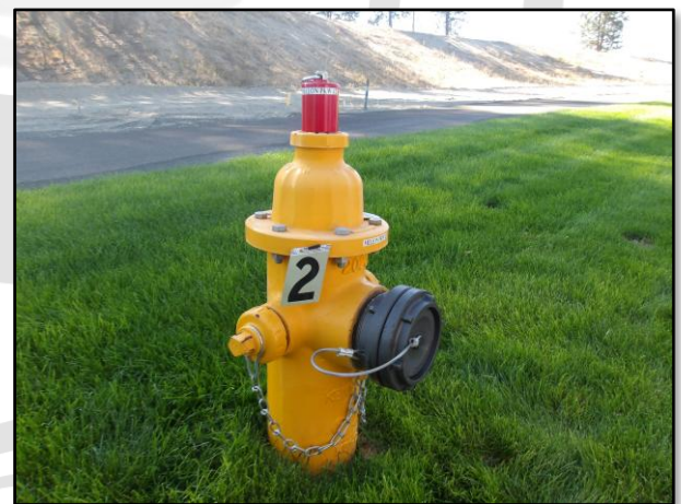
Locked Hydrant to Prevent Misuse
